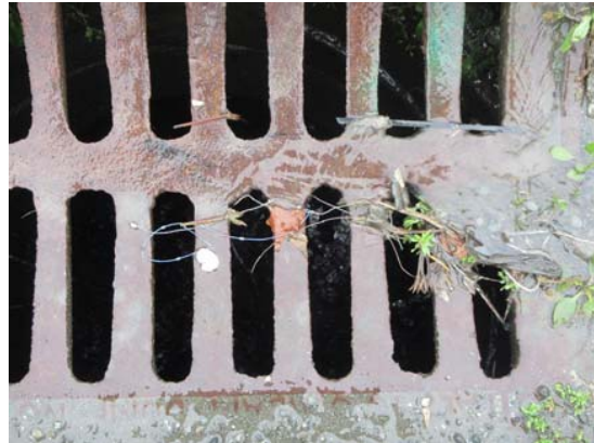
Monofilament on storm drain that empties into Ship Creek
